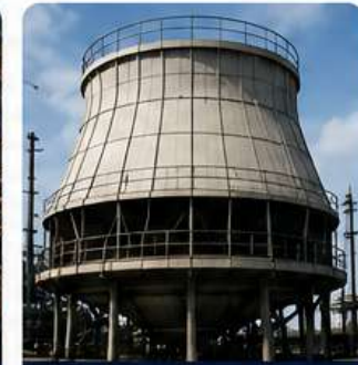
COOLING TOWER FILL
